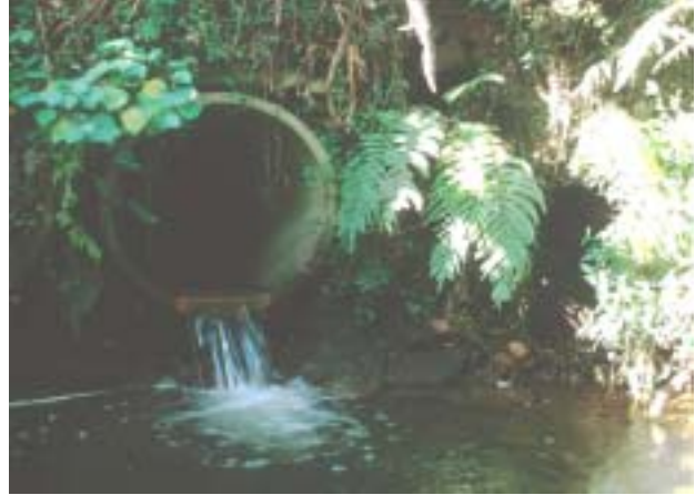
Example of a culvert that presents a barrier to fish passage
