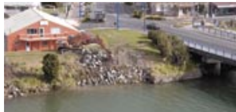
Work on rock bank lining on the Waitara River ensures the flood protection scheme is in top order.
