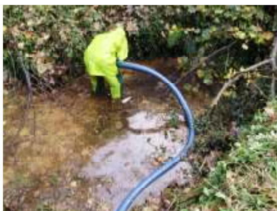
The cleanup of the discharge from Caltex, Stratford
