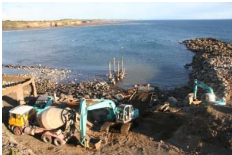
Work being carried out for the construction of the Opunake Bay boat ramp
