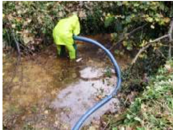
The cleanup of the discharge from Clatex, Stratford
