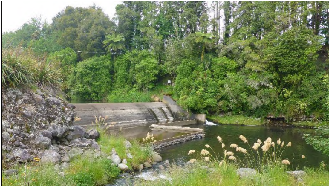
Figure 3.1. Mixture of exotic and indigenous vegetation types at the Motukawa HEPS intake weir on the Manganui River.
